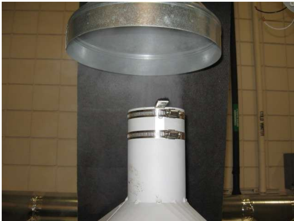
Figure 4.6. Slight back pressure over biofilter 2.
