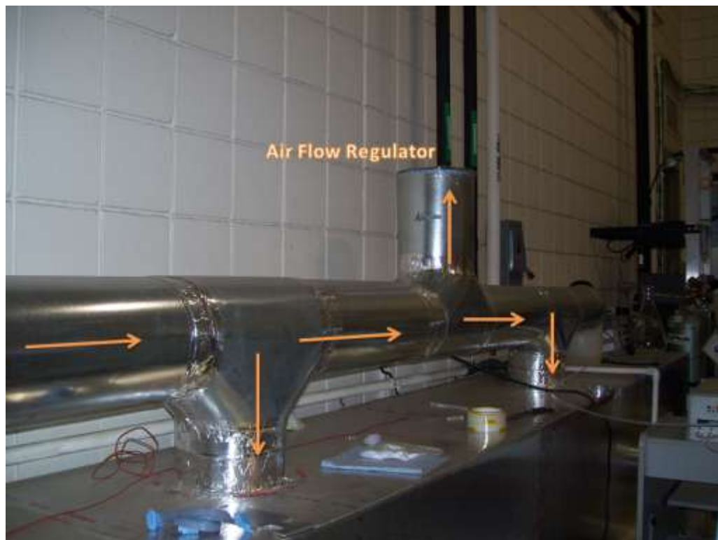
Figure 3.10. Air regulator and air delivery to the plenum.
