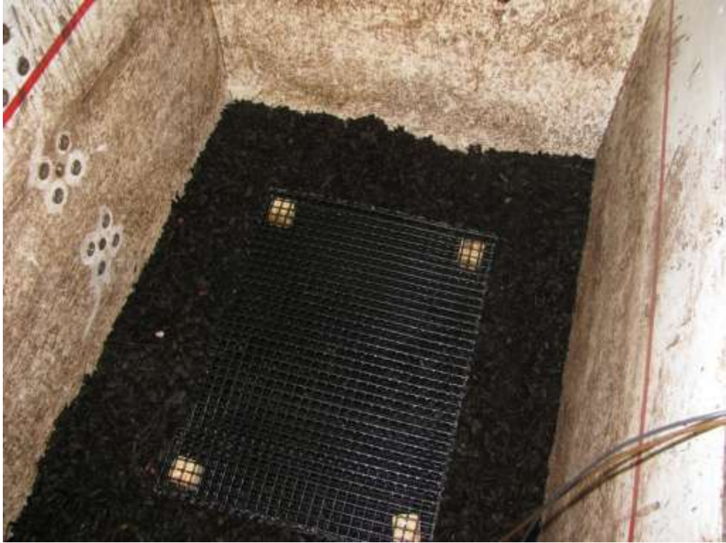
Figure A.3.2.1.1 Grids installed in the lower position of the biofilter.
