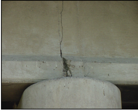
Figure 1.6 Severely Cracked Beam ends at continuity diaphragm
