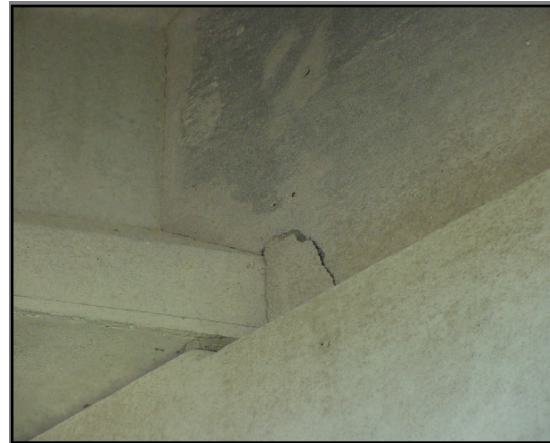
Figure 1.7 Cracking at the beam and Diaphragm intersection
