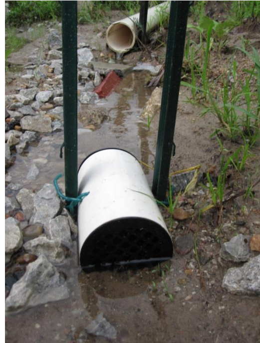
Figure 4-18 Filter Trench Effluent Sampler Deployment Unit
