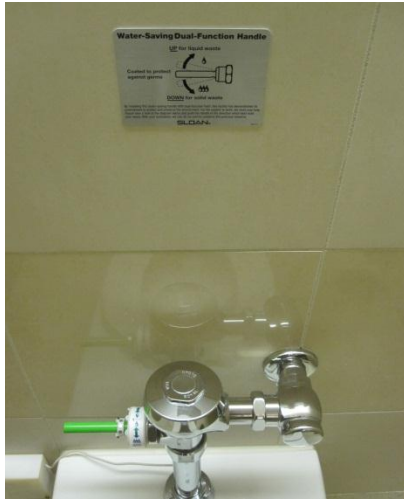
Figure 26: Instructional wall plate as installed in City Hall 1
