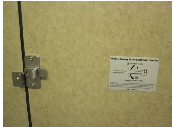
Figure 27: Instructional wall plate as installed in City Hall 2
