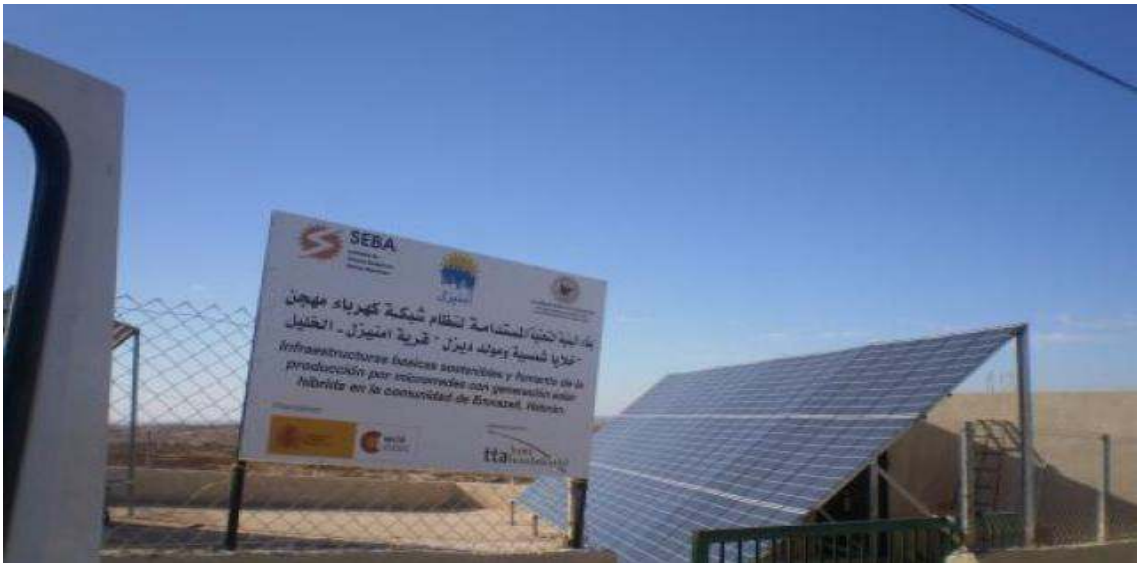
Figure (3.4): Photovoltaic solar energy panels in Amnazel Village
