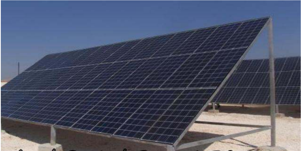
Figure (3.3): Photovoltaic solar energy panels in Atouf Village
