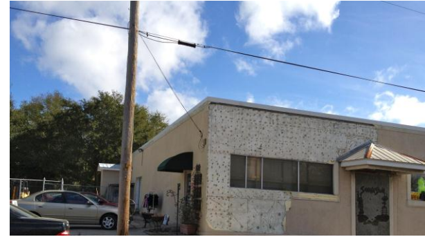
Figure A-26. Poor Façade Conditions
