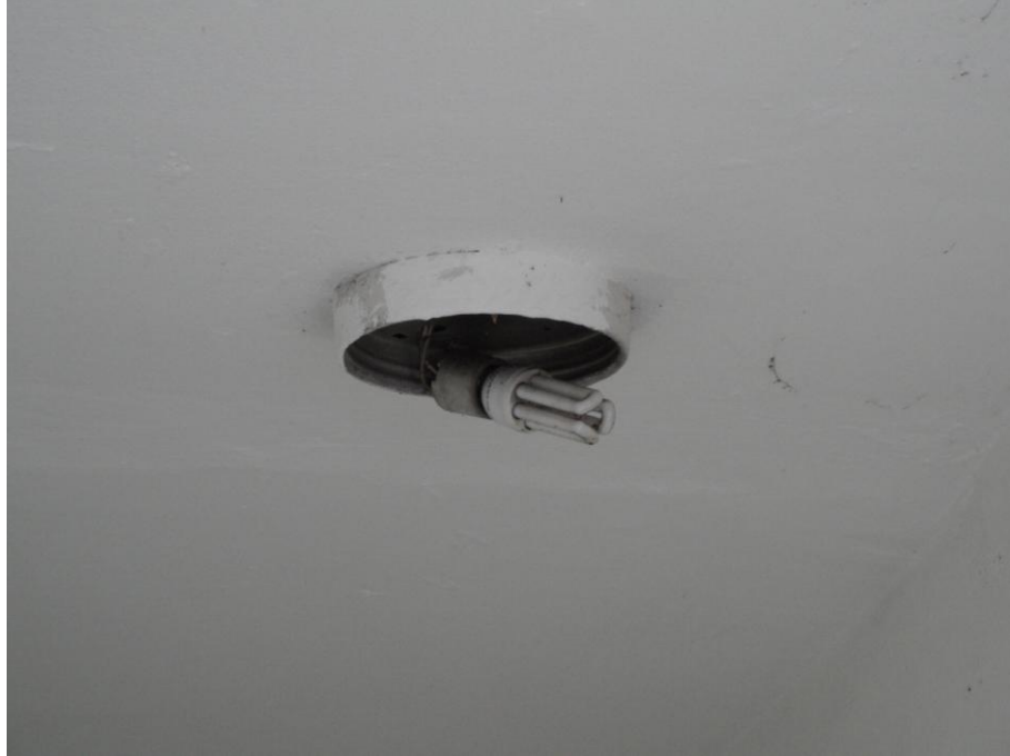
Figure 4-44. Broken automatic sensor light. Photograph by author.
