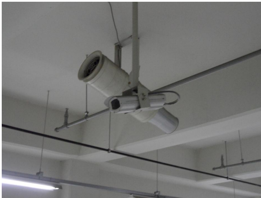
Figure 4-9. CCTV camera installed in underground parking lot. Photograph by author.
