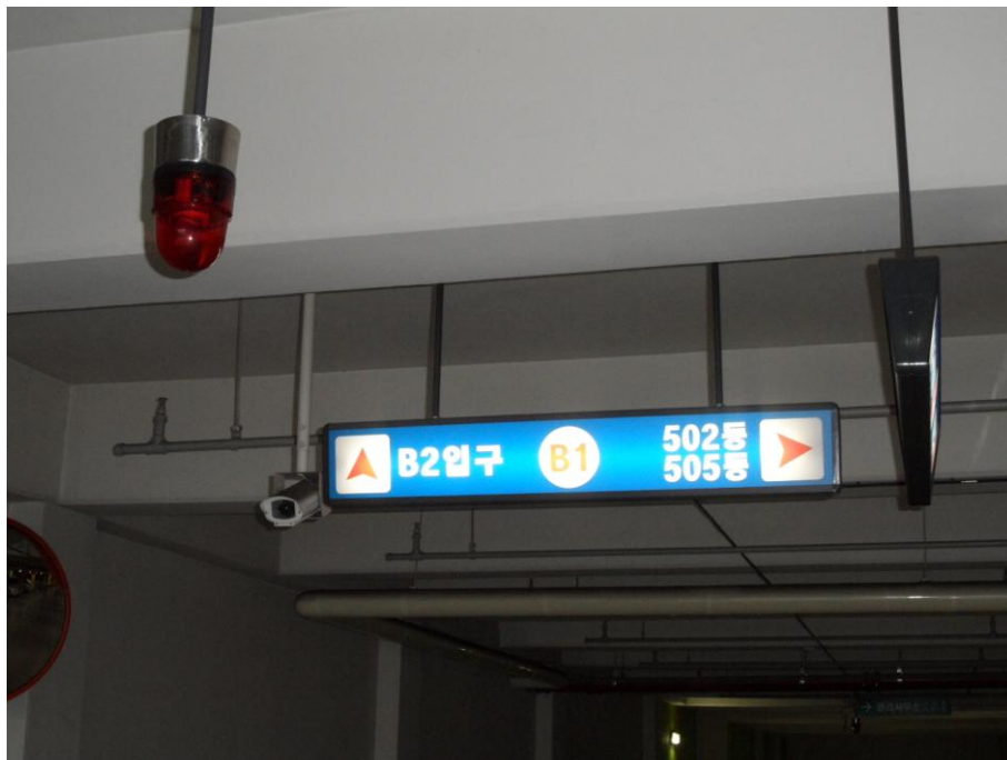
Figure 4-7. Direction signs and caution alarm at underground parking lot. Photograph by author.
