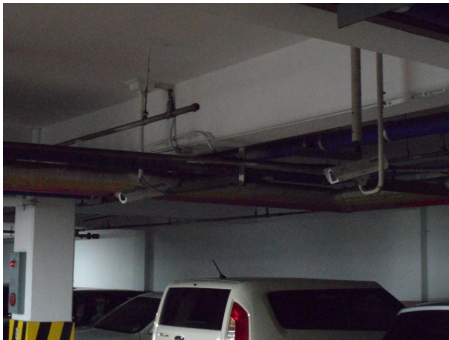
Figure 4-41. CCTV cameras installed in underground parking lot. Photograph by author.
