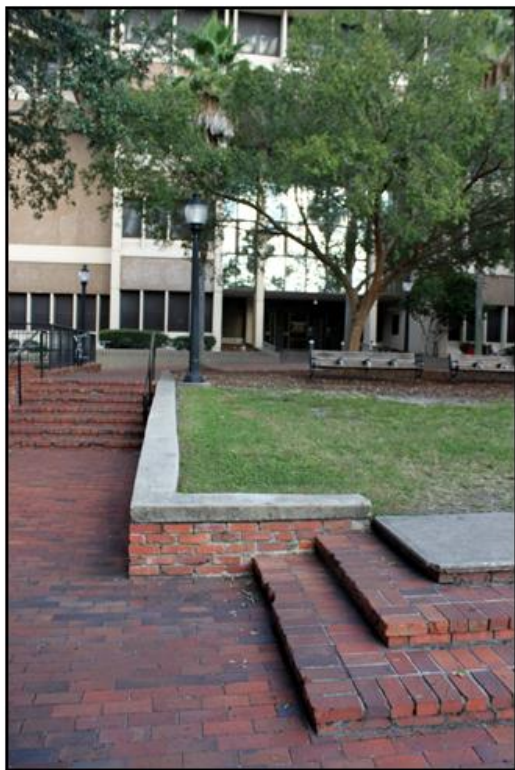
Figure 4-6. Brick ledging in Bo Diddley Community Plaza.
