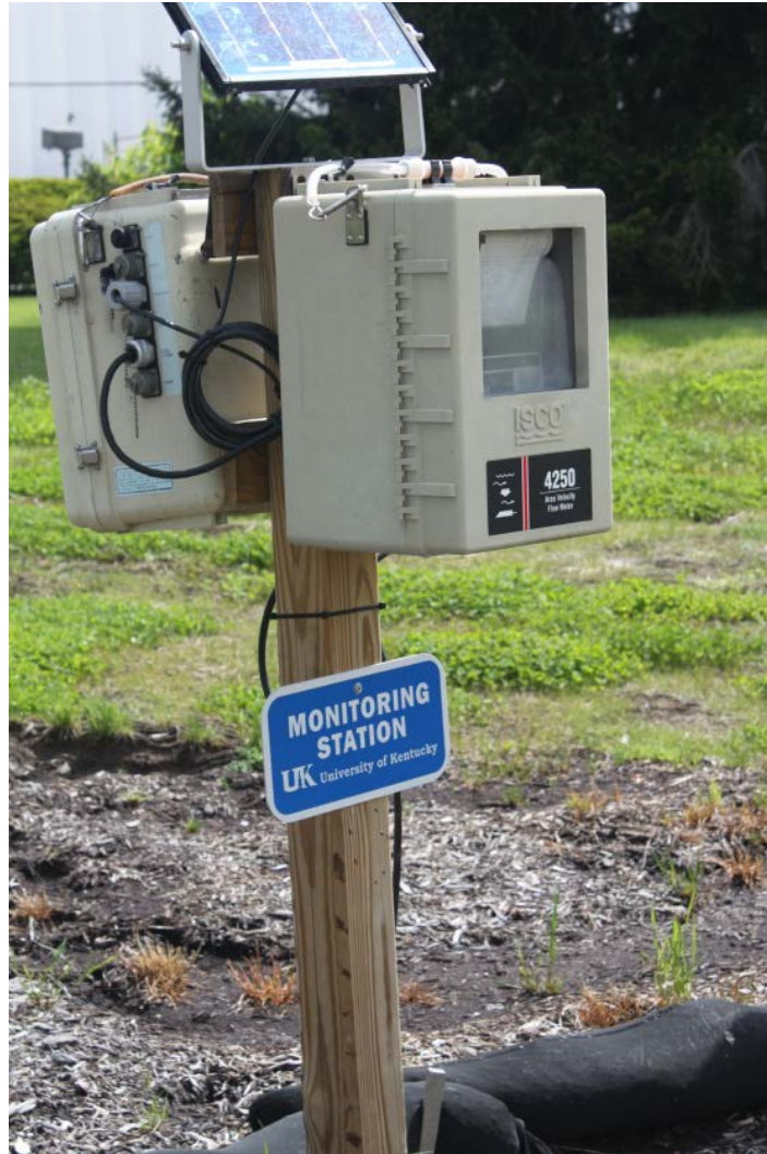
Figure 3.7. Flow meters were used to determine stormwater inflow rates through the two inlet pipes.
