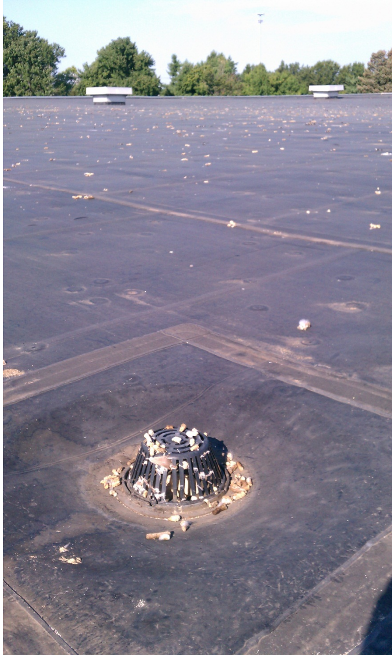
Figure 3.3. Goose feathers and droppings at the roof drain of the Coca-Cola Refreshments USA, Inc. warehouse rooftop.
