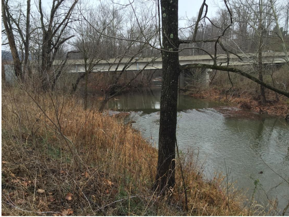
Figure A.19: Upstream view of Site ID 9: USGS gage 03250100 North Fork Triplet (HLR 9).
