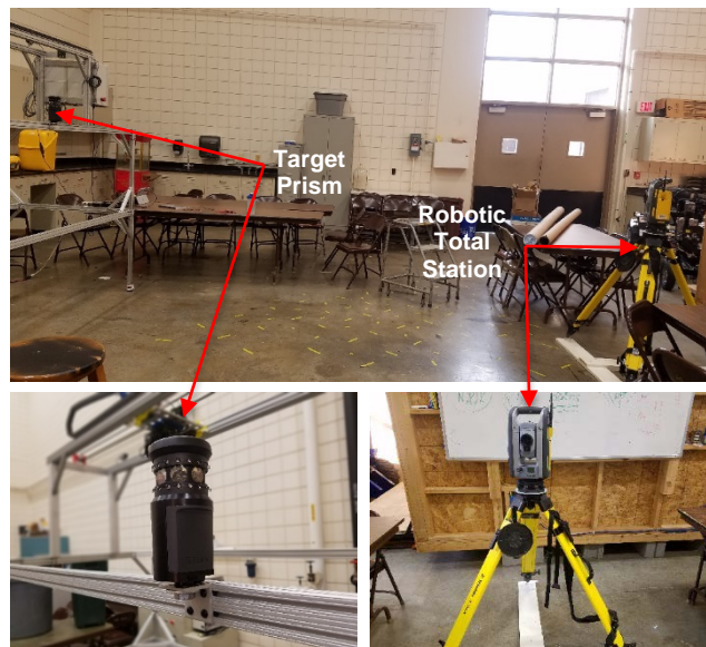
Figure 2-6: Validation of the linear motion system performance using a robotic total station and target prism.
