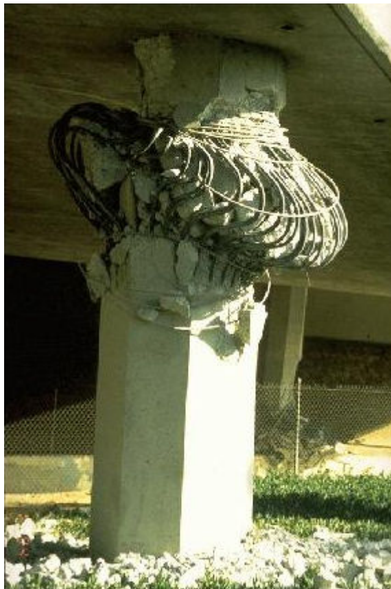
Figure 3-1. Plastic deformation of a bridge concrete column during the 1994 Northridge earthquake (Image Credit: NOAA/NGDC, M. Celebi, U.S. Geological Survey)
