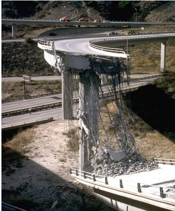
Figure 3-2. A superstructure failure during the 1994 Northridge earthquake (Image Credit: www.usgs.org )
