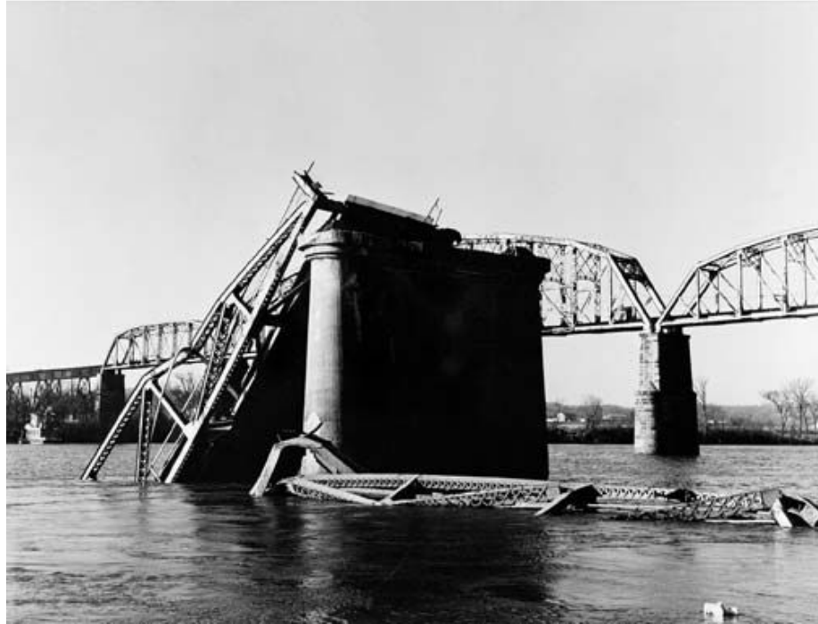
Figure 2-3. Silver Bridge failure over the Ohio River caused the death of 46 people in 1967 (Image credit: http://www.pbs.org/ )
