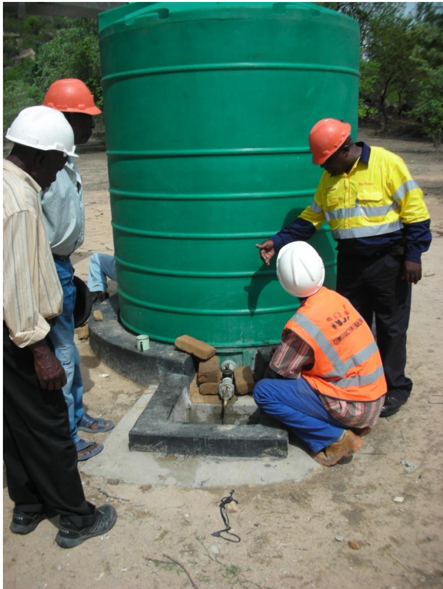
Mr Mudondo providing advice on the installation of a water tank at the site.
