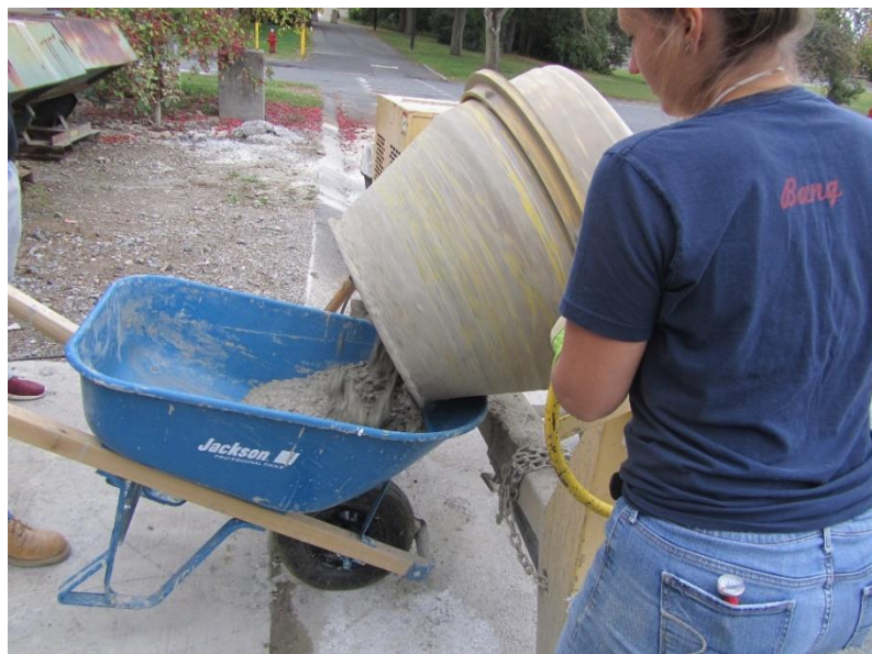
Figure 4-3: Removal of Concrete from the Machine Mixer in Preparation for Testing and Casting
