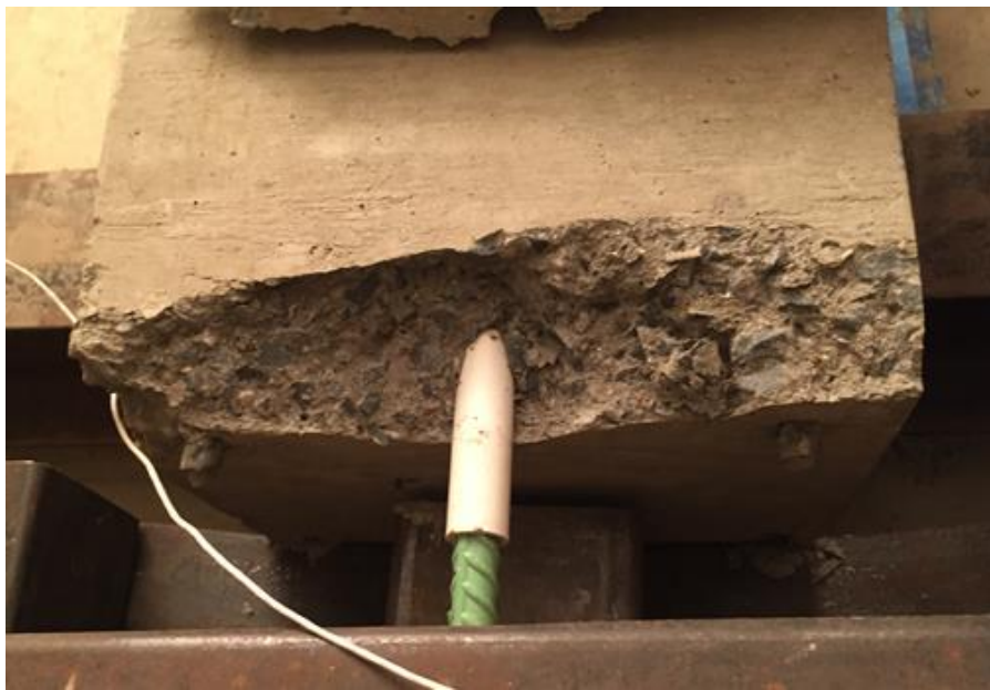
Figure 5-15: Concrete Cracking of Test Specimen 15-HD-6
