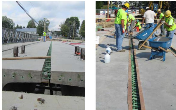
Figure 1-1: Closure pours in a Massachusetts precast bulb-tee bridge using UHPC (pictures courtesy of S. Brena)
