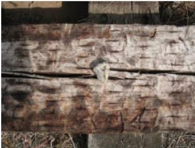
Figure 2.3 Underside of a conventional wood tie removed from service showing indentations from ballast particles. (FRA Task Order 225)
