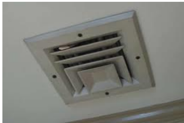
Figure 4.4 : The Vents of HVAC
