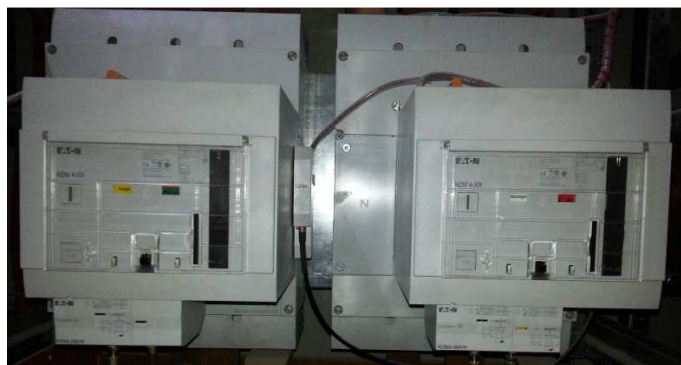
Figure(3.6): Indoor of ATS board in electrical distribution board
