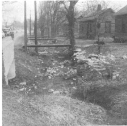
This open sewer west of Providence Road caused many health, sanitation and flooding problems.
