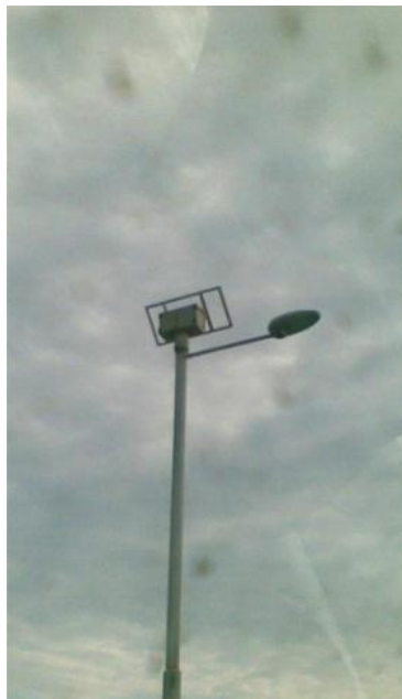
Figure 3.11: Fixed Solar Panels for Lighting Gaza Valley Bridge
