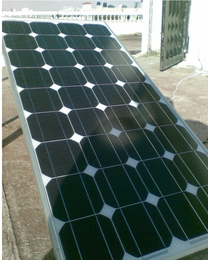
Figure 5.3: Mounted PV Module on roof building
