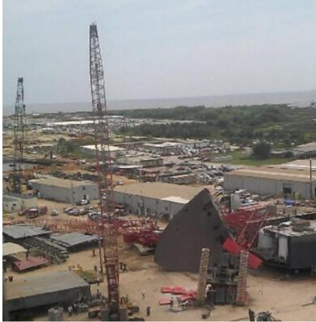
Figure 6: Tandem Lift Accident [4].
