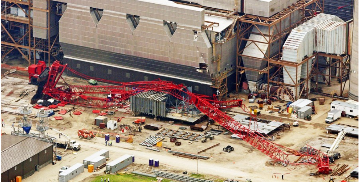
Figure 7: Crawler Crane Tip-Over Accident [23].
