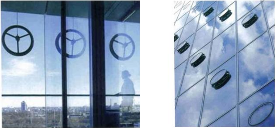
Figure 5: Examples of ventilation ports in the Uptown München tower
