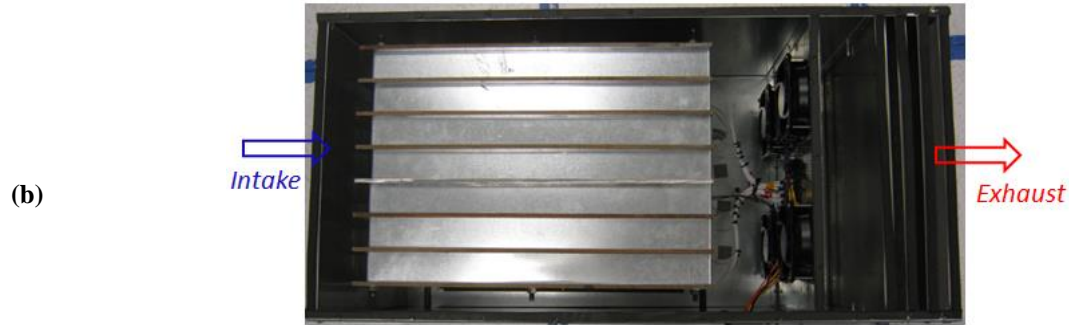
Figure 2.8: Chassis layout: (a) Drawing (dimensions in inch); (b) Photograph from the top (cover removed).
