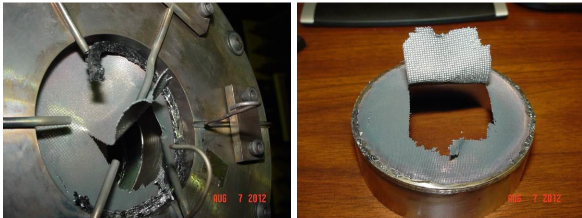
Figure 30 Second Screen Flow Conditioner Failure
