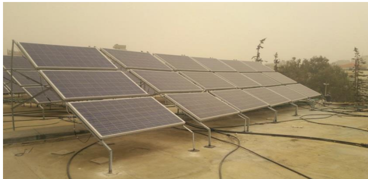
Figure 2.6: Solar energy project in Al-Naser hospital
