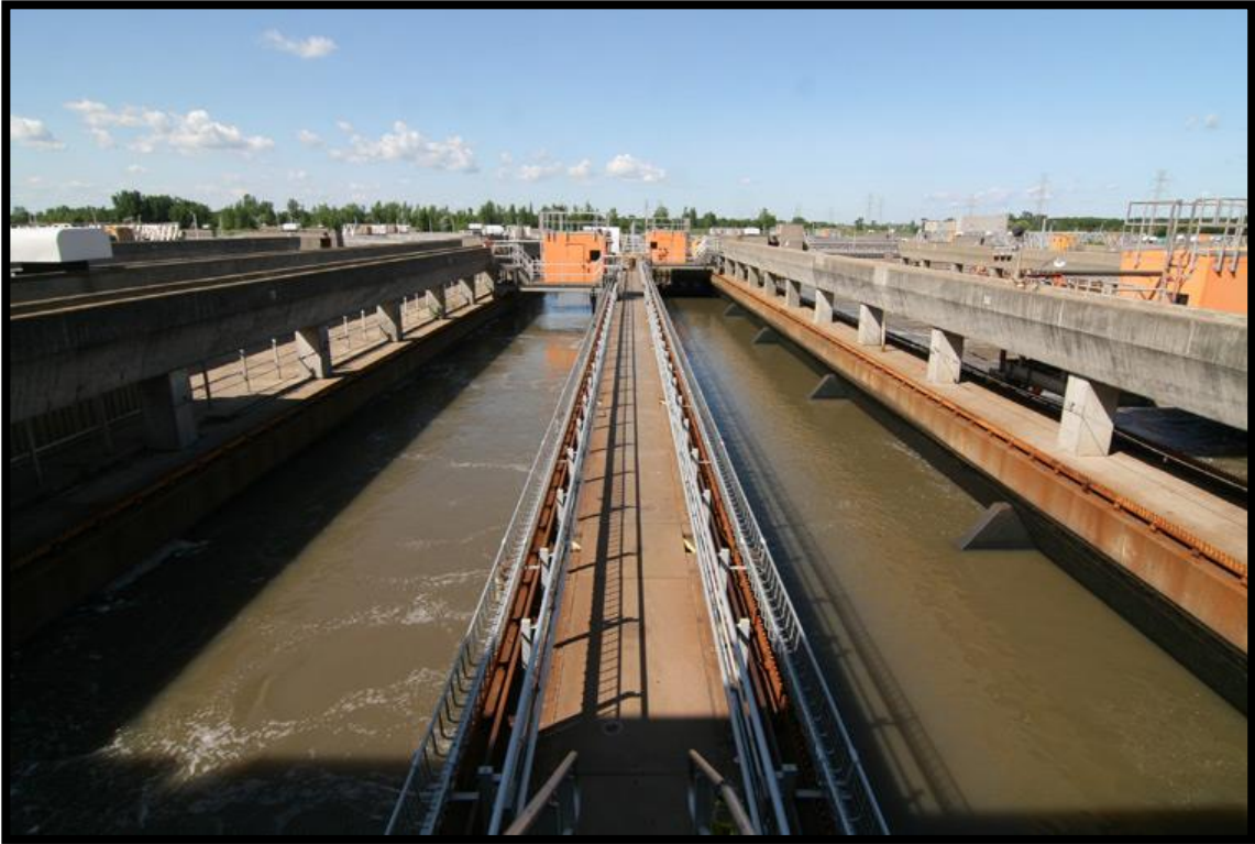
Figure (2.2): Grit removal channel.
