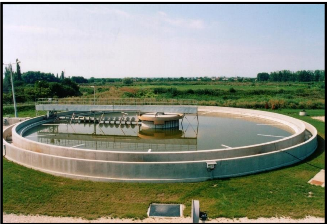
Figure (2.3): Sedimentation tanks.
