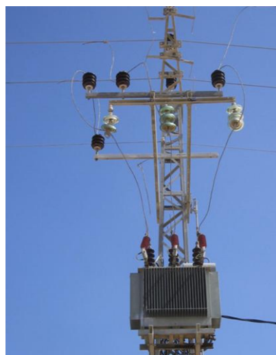
Figure 3.3: One of the distribution transformers used by GEDCO
