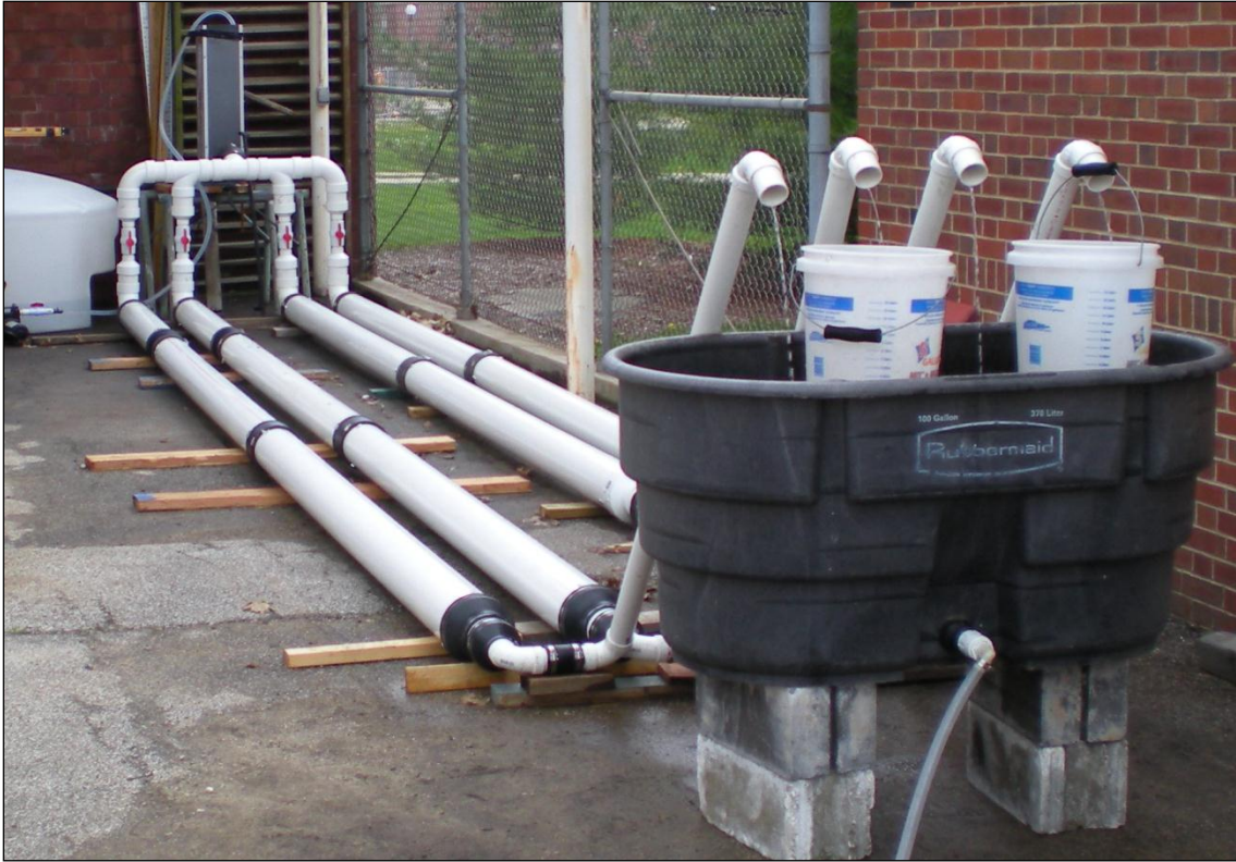
Figure 5.5 Four-Column Reactor used in Column Reactor Experiments.
