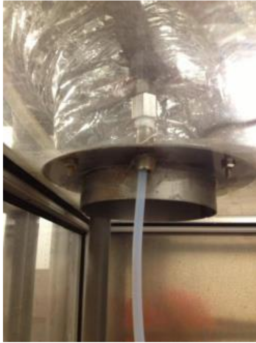
Figure D.1: Picture showing injection tube directed into sampling port.
