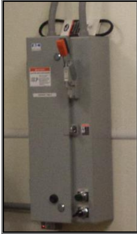
Figure G.6: Power switch for Animal Space Exhaust Unit.
