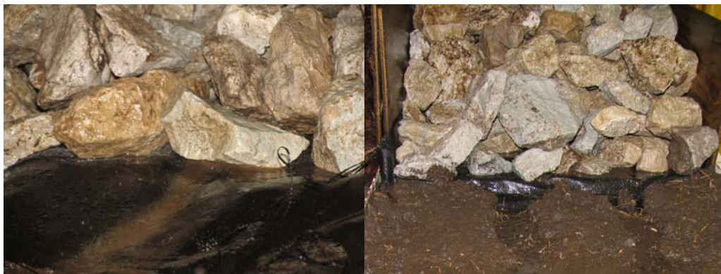
Figure 5.14. The concentration of flows and the resulting rill formation in riprap berms.
