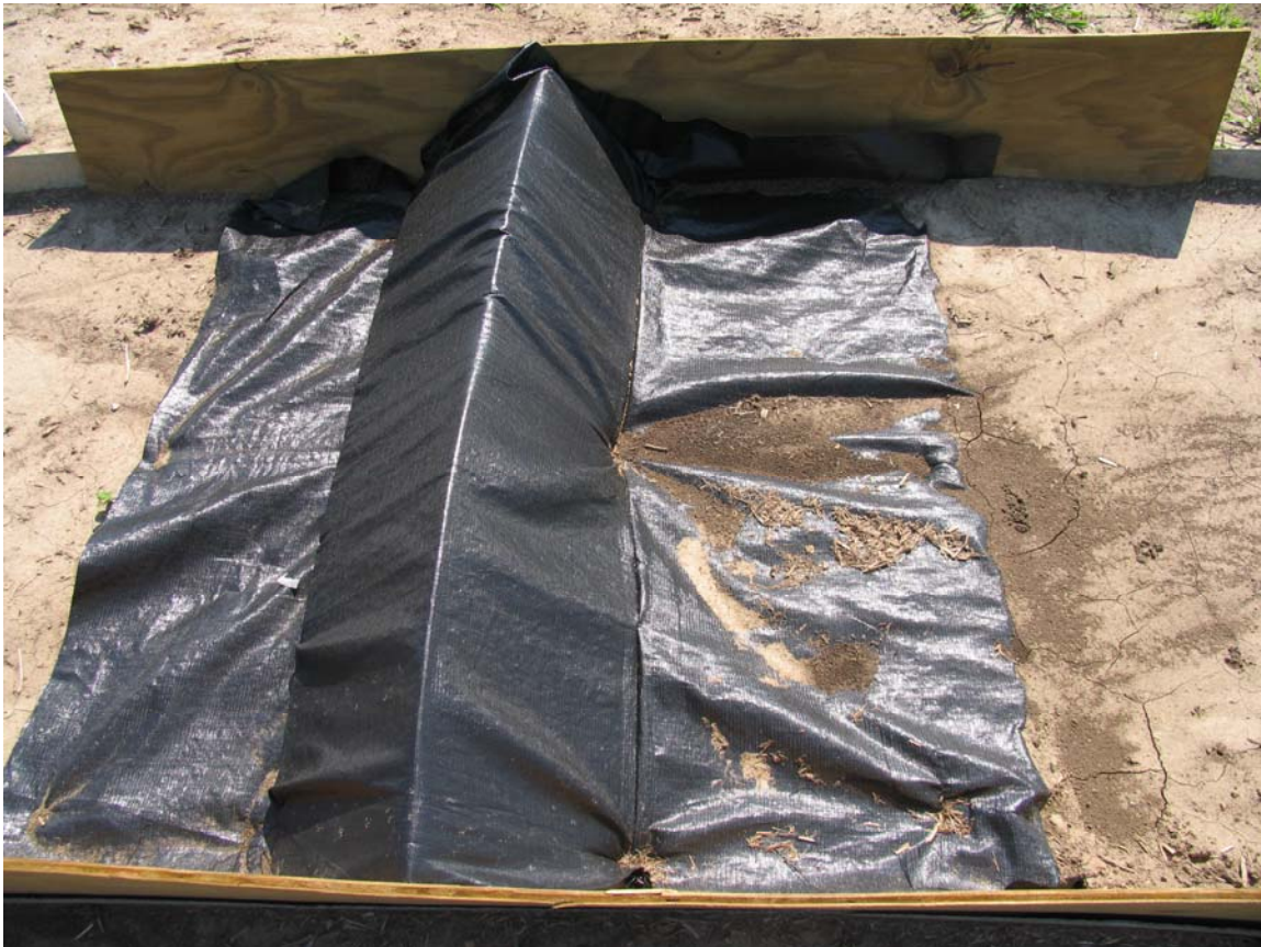
Figure 4.7. Foam dike at field site.
