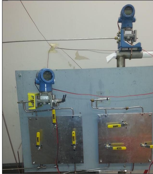
Figure 3.10 Rosemount Gage and Differential Transmitters
