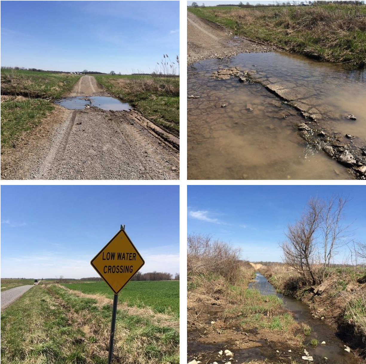
Figure 4.14: Franklin LWC site, crossing surface, sediment deposition downstream, signage (clockwise).
