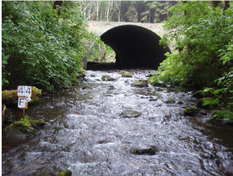
Figure 3.4: Culvert for AOP, which mimics the natural bedstream (from Barnard et al. 2013).
