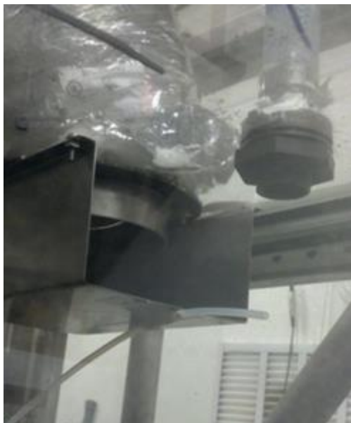
Figure E.2. Injection point taped next to ventilation inlet and recirculation return.
