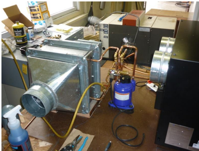
Figure 2-14. View of exhaust ductwork and heat exchanger, compressor, reversing valve, and ERV.
