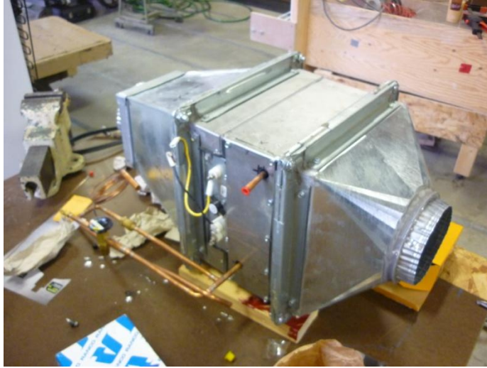
Figure 2-13. Ductwork surrounding supply heat exchanger.
