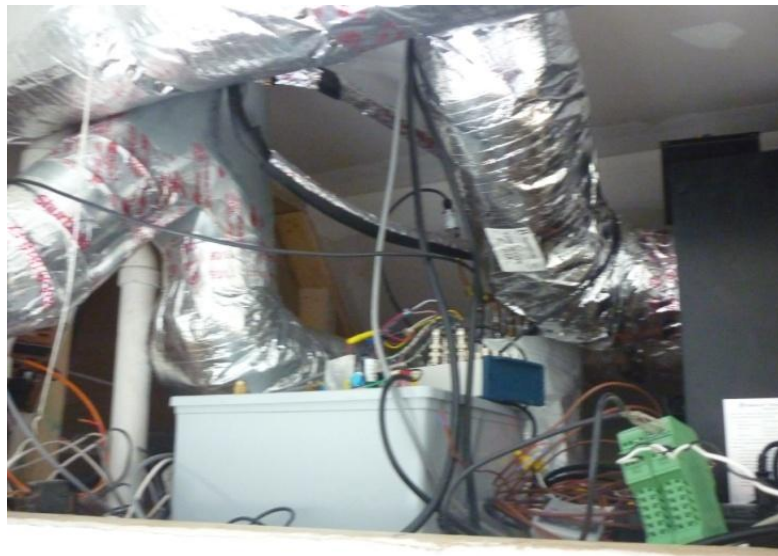
Figure 2-16. View of installed HVAC system with duct insulation and control boxes.
