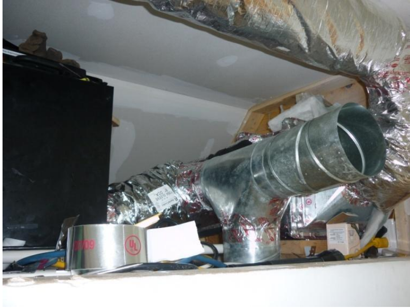
Figure 2-17. View of installed HVAC system towards return and supply ducts.
