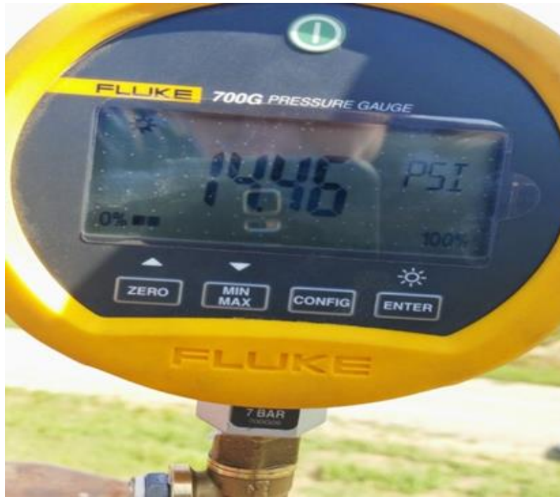
Figure 13. Measurement of Discharge Pressure of a Relift Pumping Plant using a Digital Fluke Pressure Gauge.
