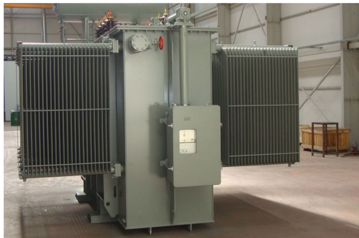
Figure 6. 1 MVA transformer with radiator banks for additional cooling [3]
