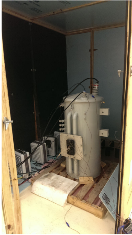
Figure 26: 50 kVA thermosiphon-transformer assembly in testing chamber
