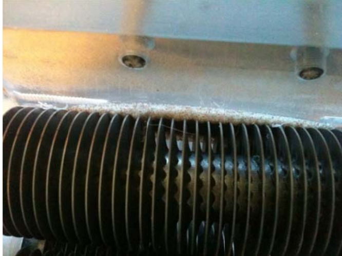
Figure 5: Finned Tube Fusing with Polycarbonate and Sand Leading to Obstructions
