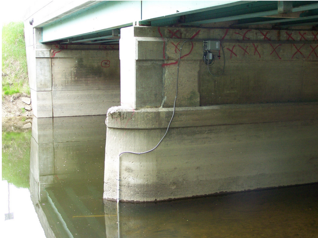
Figure 5.6. Bridge with a monitoring system in Flint, MI. Data is collected and transmitted to a remote computer once per hour. System and photo by Fondriest Environmental [60].
