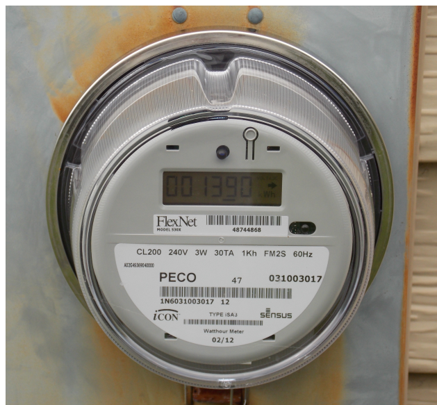
Figure 3.1. Smart meter installed in the state of Pennsylvania in 2012.
