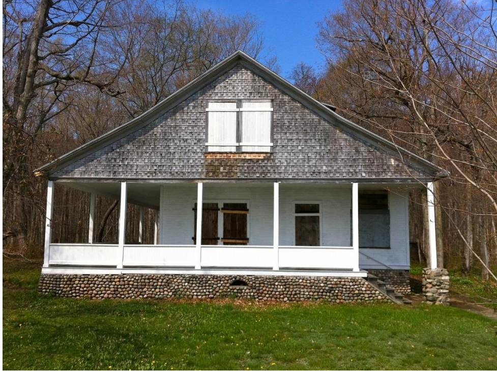
Figure 27. The Katie Shepard Hotel, an example of historic preservation on Cottage Row. Photograph by Kimberly Mann, Historic Architect, Sleeping Bear Dunes National Lakeshore, 2011.
