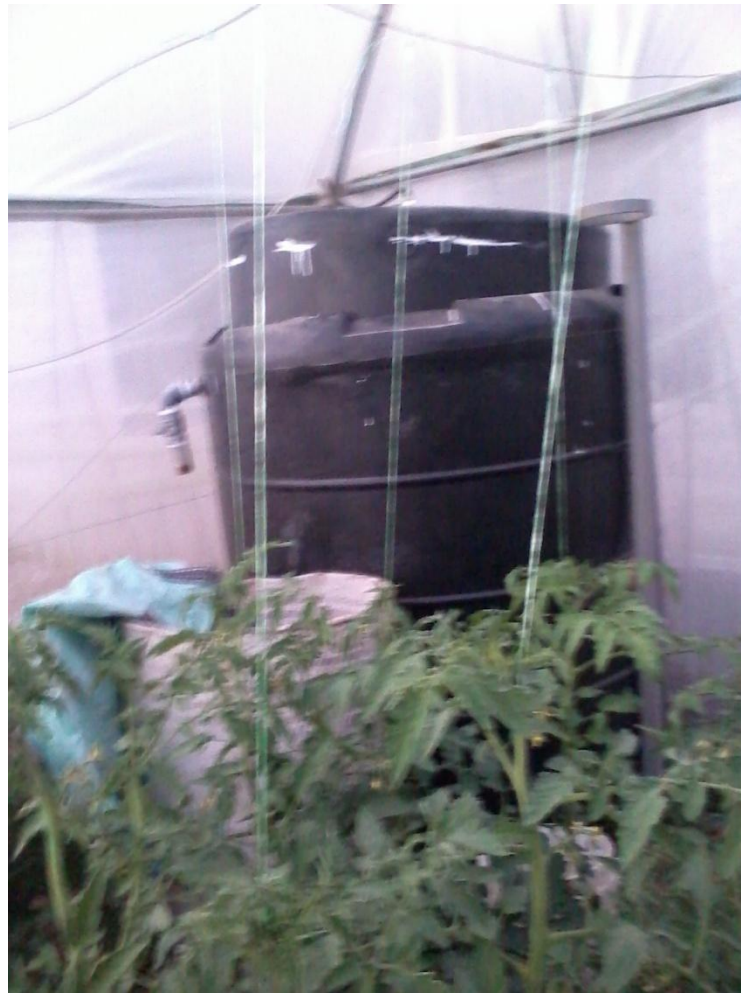
Figure 6: The biogas unit inside the greenhouse
