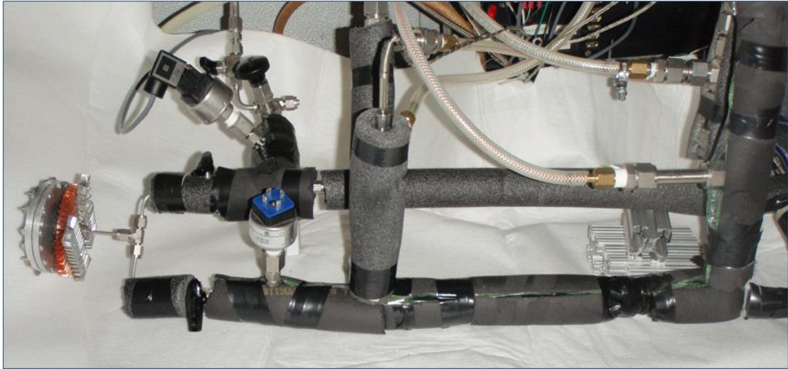
Figure 4.3 Photograph of the experimental facility. The adsorbent bed is in the lower left-hand corner. The ball valves are the black handled connections next to the insulation.
