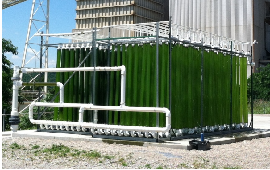
Figure 2.17: Duke Energy, East Bend Station pilot reactor; 20,000 L.
