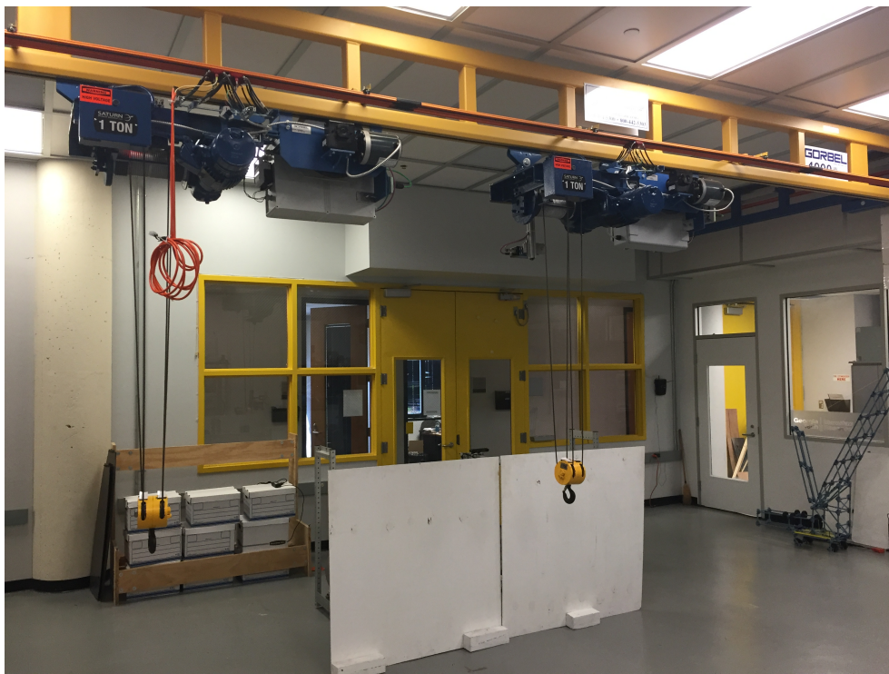
Figure 1: Two-Ton Dual-Hoist Bridge Crane
