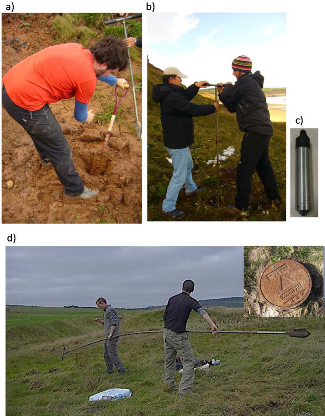
Figure 3.13 Piezometer installation by hand auger: a) preparing the borehole for Casagrande piezometer; b) Using the hand auger to drill a borehole of about 4 inch in diameter; c) Standpipe piezometer tip; d) The long extendable steel rods of hand auger is about 6 m.
