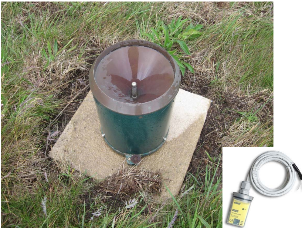
Figure 3.14 A tipping bucket rain gauge and its data logger on top of the cliff
