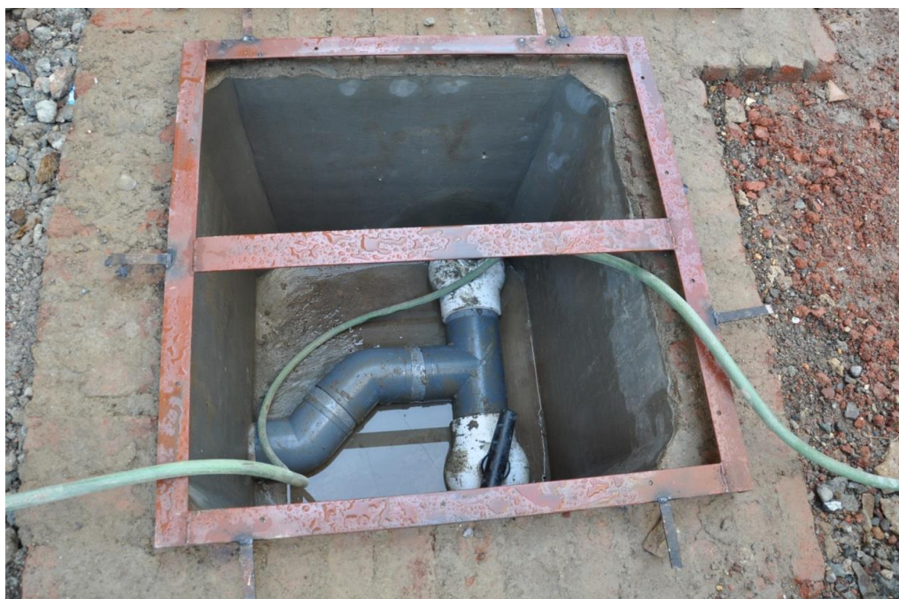
Figure 6.5: First flush valve to clean the system (Source: Author)
