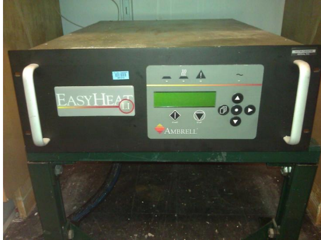
Figure 76. 10 kW EasyHeat LI power supply used for induction heating
