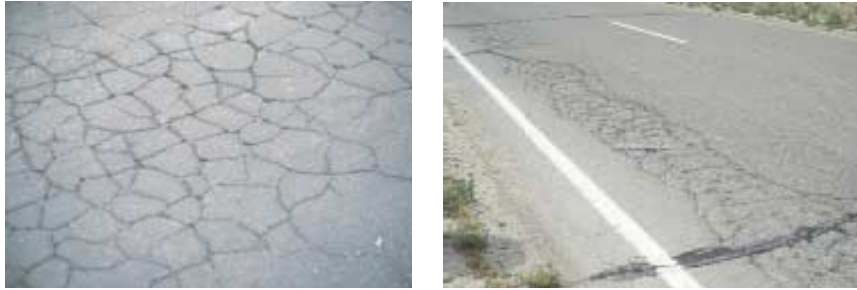
Figure 2.2 High severity fatigue cracking [6]
