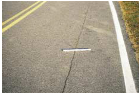
Figure 2.4 High severity longitudinal cracking [6]
