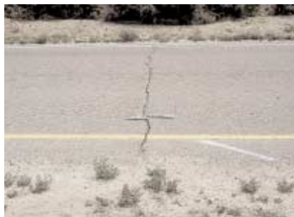
Figure 2.7 High severity transverse cracking [6]
