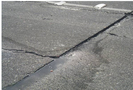
Figure 2.12 High severity faulting [6]
