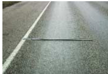
Figure 2.6 High severity rut [6]
