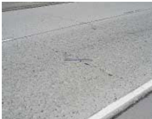
Figure 2.9 High severity transverse cracking [6]
