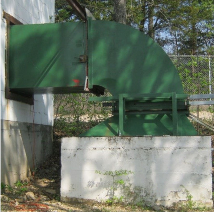
Figure 3.6 Missouri S&T surface main fan ventilation system elbow
