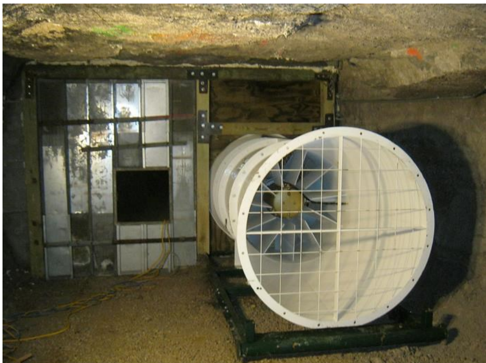
Figure 3.10 Booster fan bulkhead- front view
