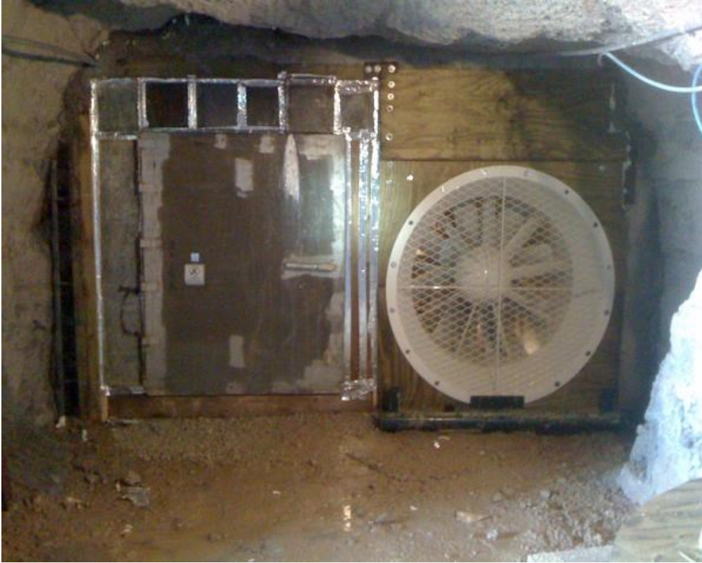
Figure 3.11 Booster fan bulkhead- rear view
