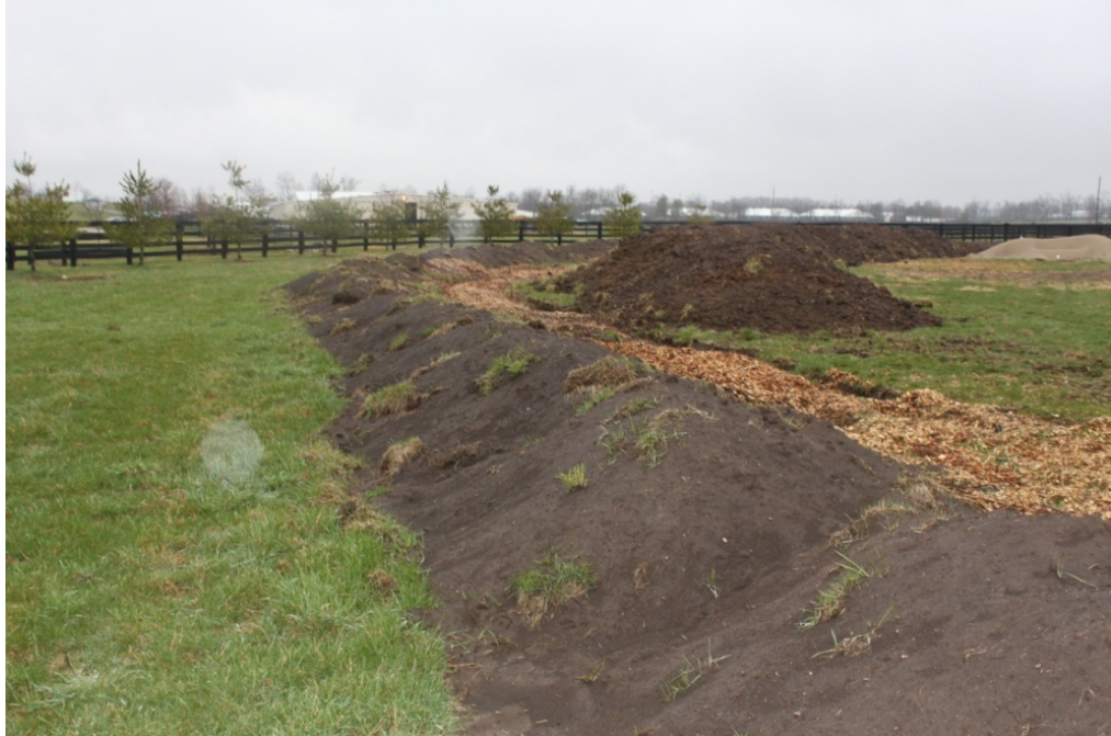
Figure 2.14: Modified Contour Weep Berm Wood Chip Trench with Excavated Soil Down-gradient for Berm Construction and Extra Soil Up-gradient for Contour Weep Berm Construction.
