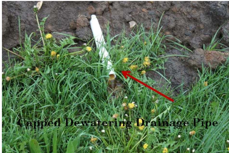
Figure 2.12: Drainage Pipe for Completely Dewatering the Contour Weep Berms.
