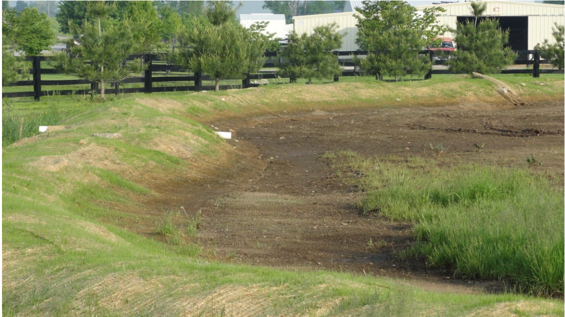
Figure 2.17: Modified contour weep berm system with erosion matting and seed after construction.
