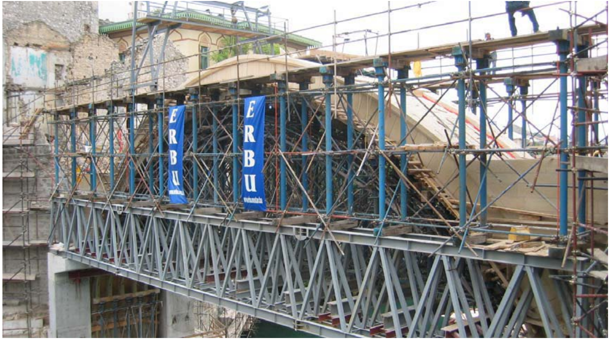
Figure 12: New Old Bridge under reconstruction, with banners naming the construction firm and donors hung onto scaffolding. Source: Makaš, 2007. Used with permission.
