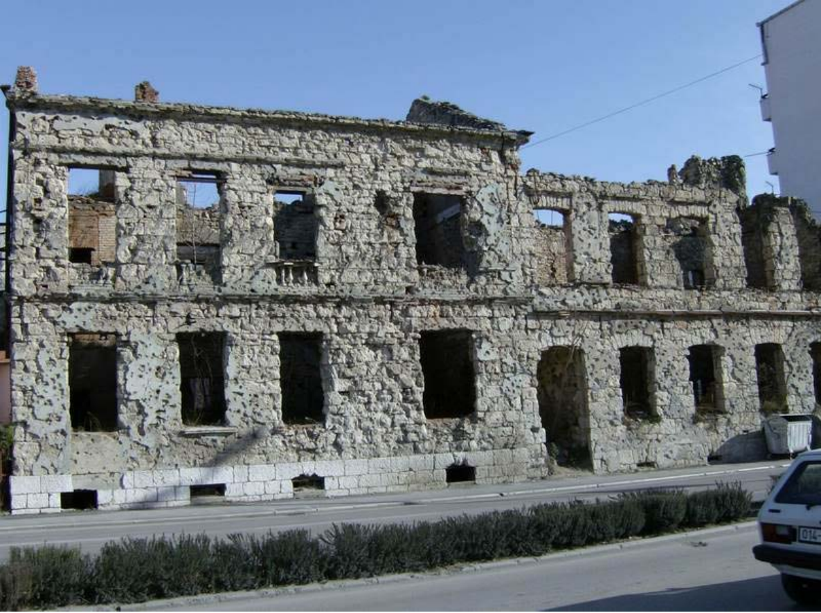
Figure 7: Damaged buildings in the city center. Source: Michael Sherman, 2007. Used with permission.
