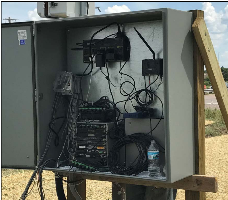
Figure 3.11 - View of Interior of Cabinet
