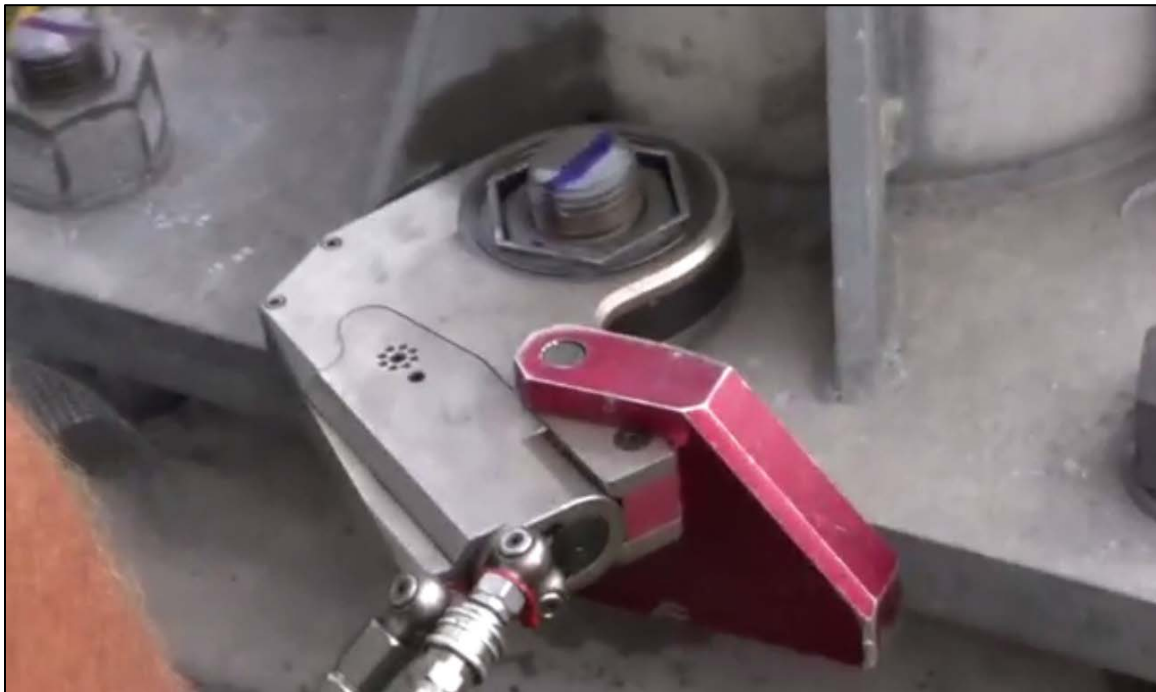
Figure 1.20 - Hydraulic Wrench Used for Maintenance Retightening
