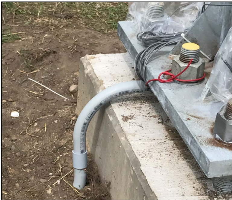
Figure 3.9 - Conduit Leading to Data Logger
