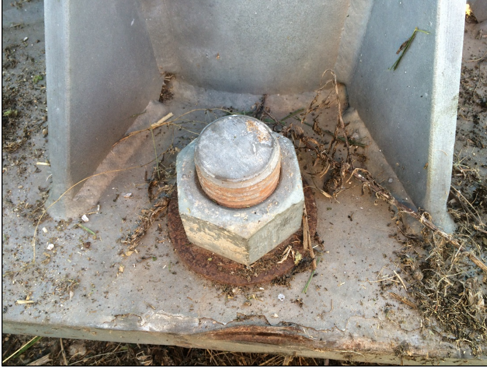
Figure 1.31 - Rusted Washers Found in District 6
