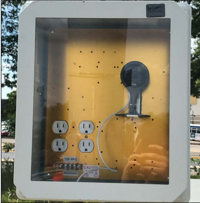
Figure 3.12 - Camera Inside Enclosure
